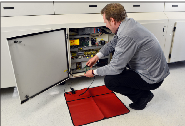
Figure 1. Proper field service ESD control.
